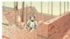
Lay the walls straight in plumb and at right angle. Make depth in shown in picture and that fit the middle part
